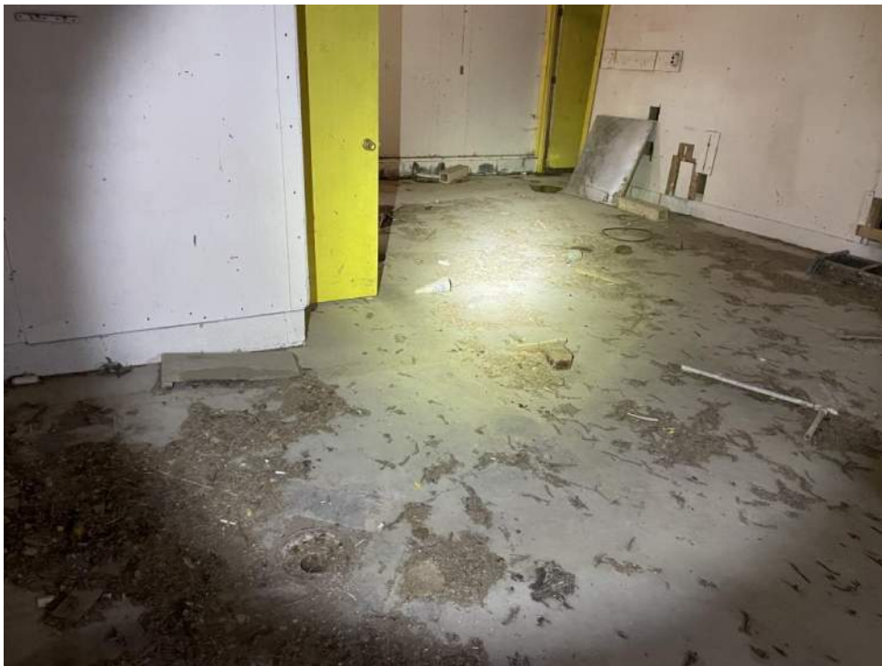
Drain noted inside central room (typical to many of the barn structures).
