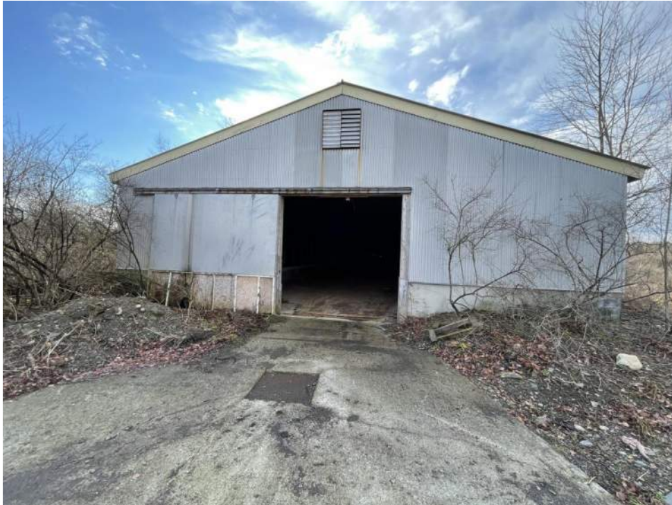
Typical view of similar barn structures present on-site with pit positioned at entrance.
