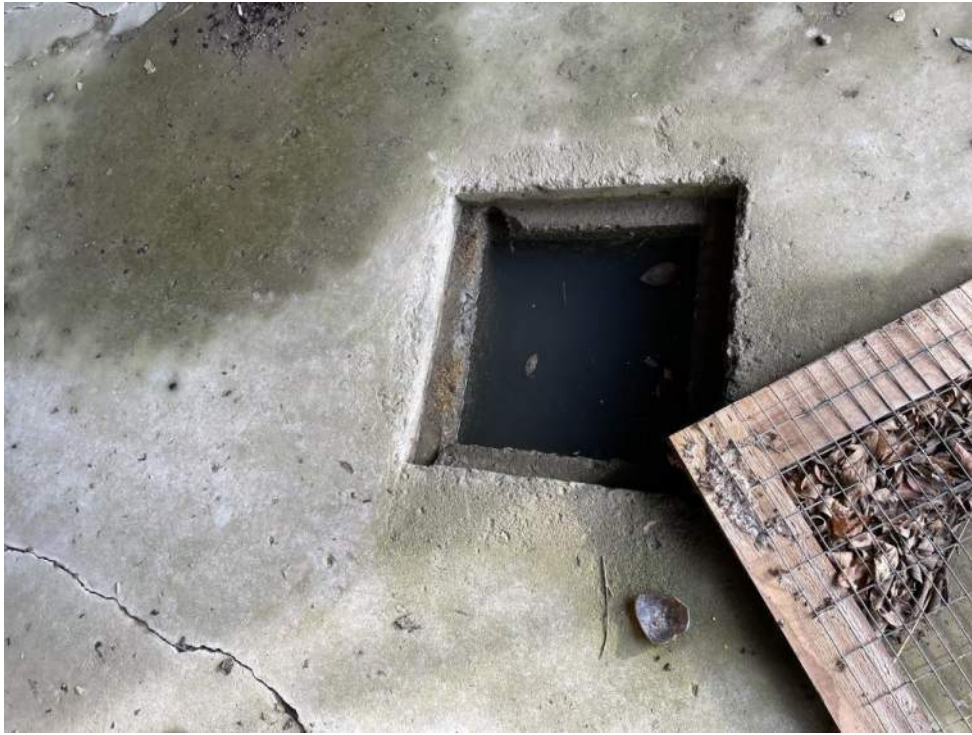
View of pit containing stormwater.
