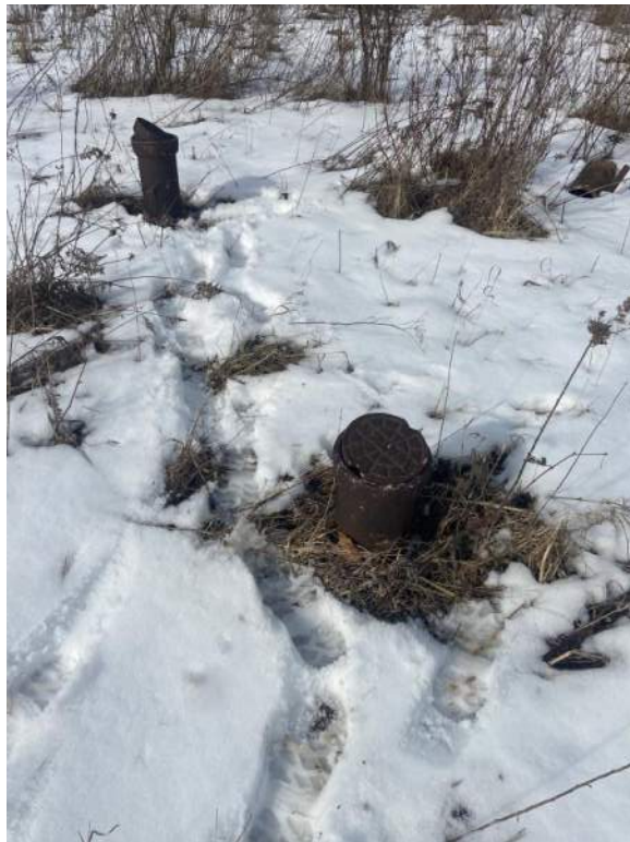
View of water line shutoff valve casings.
