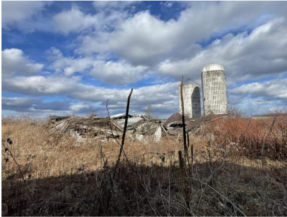
Remaining portions of structure(s) at above noted farmstead at Tucker and Aiken Road intersection. Interior portions were not inspected due to personal safety concern.
